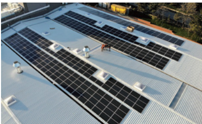
BULGARIA INDUSTRIAL&COMMERCIAL ENERGY STORAGE SYSTEM
